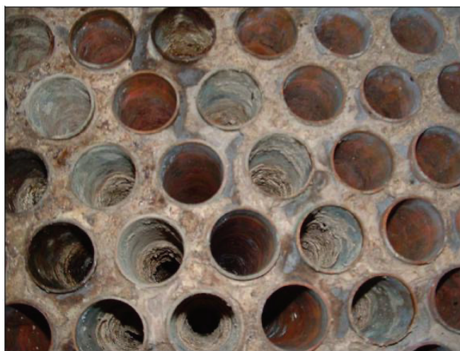
Figure 1: Equipment fouling & scaling
