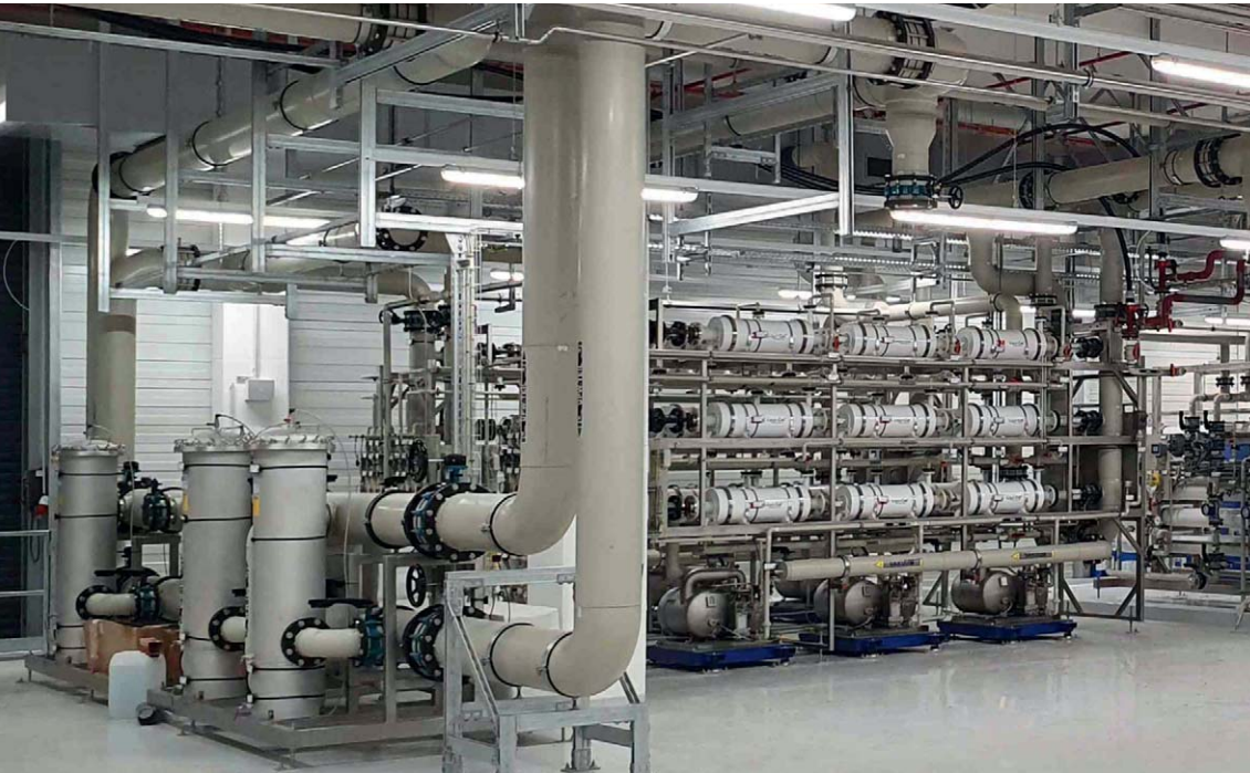
Pre-filter and membrane degasifier
