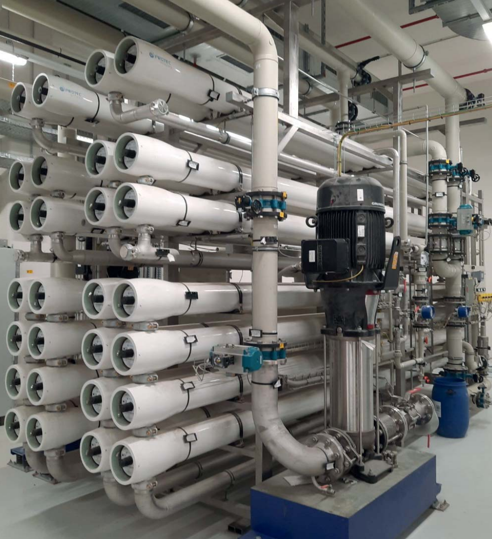
Reverse osmosis plant
