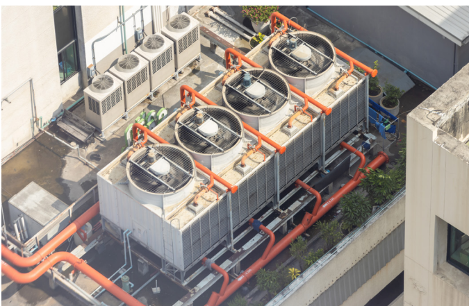
Figure 1: Open-Recirculating Cooling Tower at a Data Center Facility
